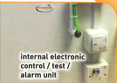
Heater cable runs inside condensate pipe through wall
